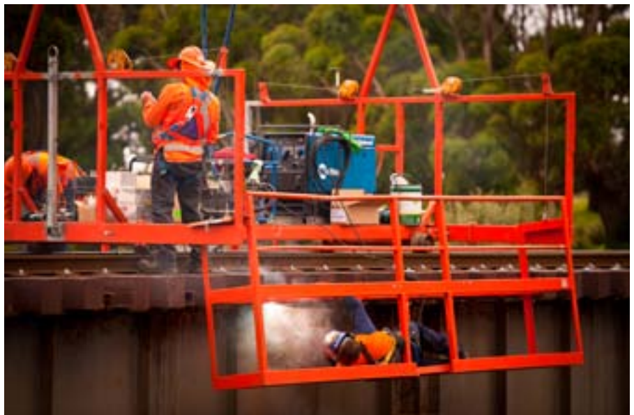
Contractors use a mobile scaffolding unit to carry out safe and rapid repairs on an open deck bridge.
