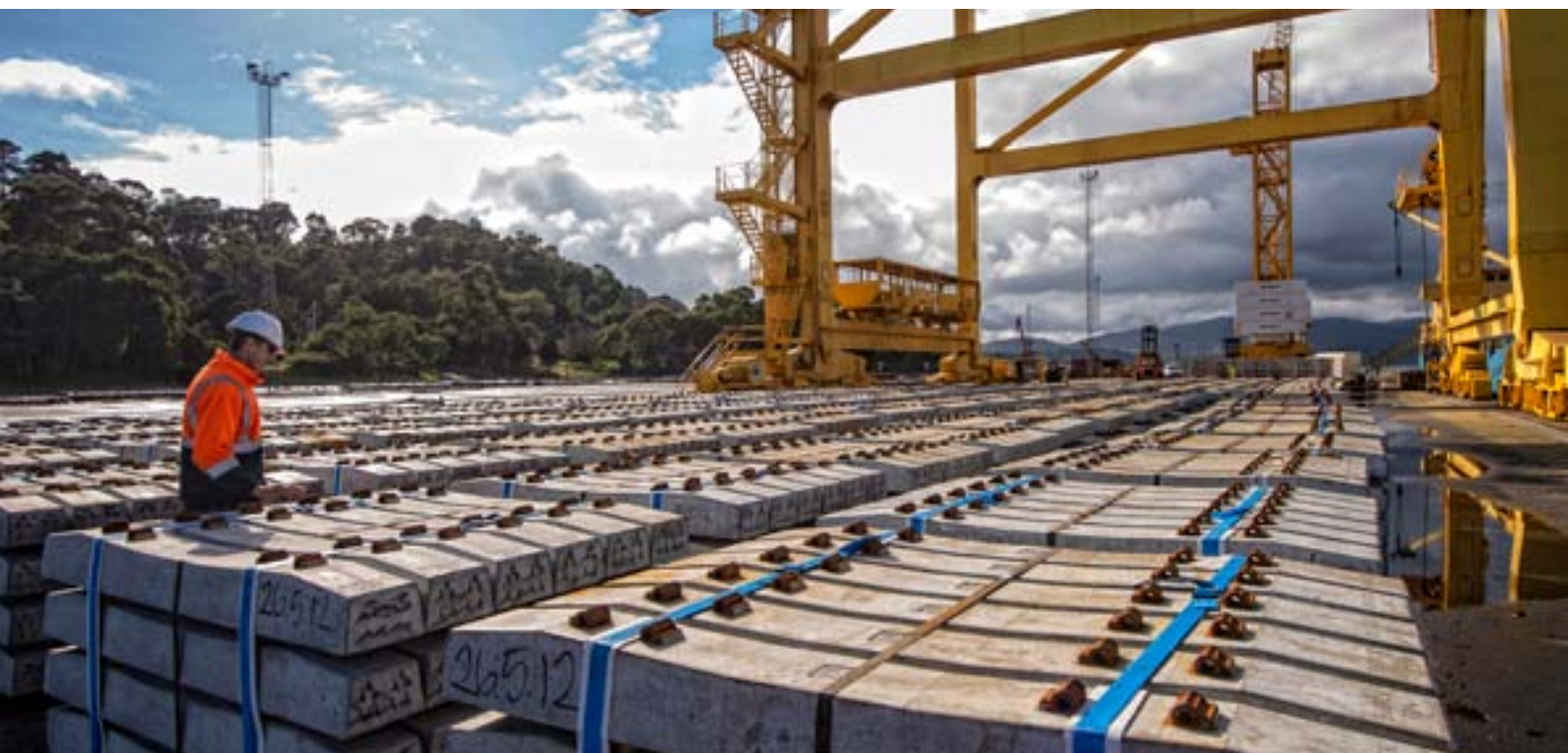
TasRail is set to commence its concrete sleeper installation program across some 70 kilometres of the rail network.
